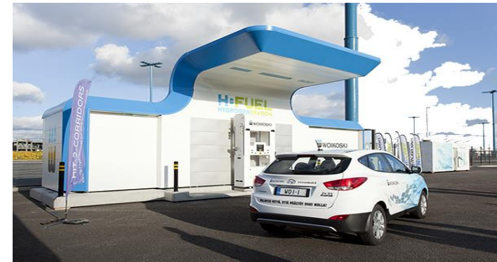
Figure 7. Hydrogen refuelling station from Woikoski [11].
